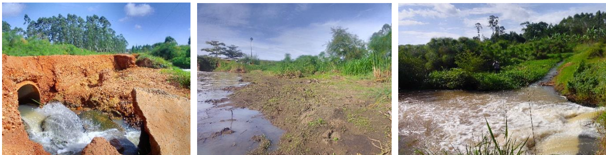
Plate 15: Destruction and erosion of part of Nyanja Road in Kijabijo (Left), flooding of the wetland (Middle-Right).
